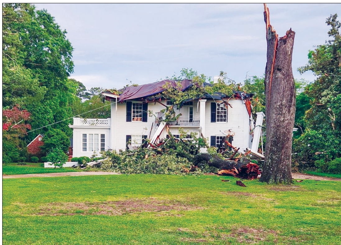
The former Powers-Beckett Home sustains damage to its front facade after a storm swept through Houston County over the weekend.
