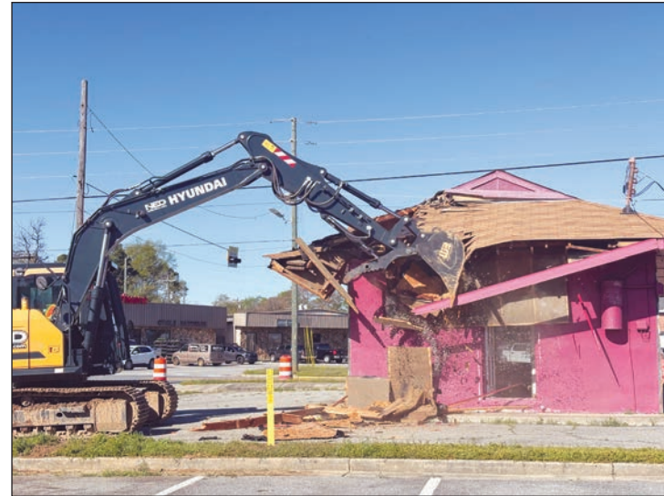
The next phase in Operation Reawaken results in demolishing the second vacant property on Commercial Circle, Tina's Barber and Style Shop.
